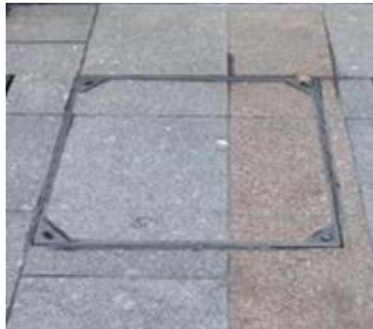
Service cover is concealed reducing visual clutter. (Courtesy of: DDS Architects)
