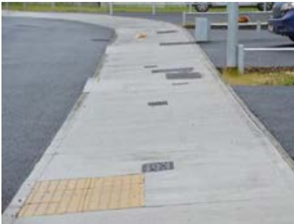
Service covers add to the visual complexity. (Courtesy of: DDS Architects)
